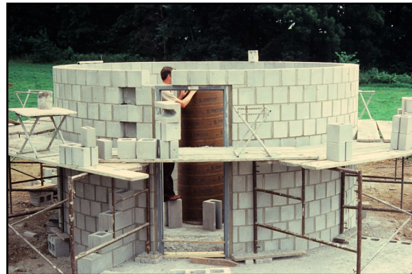
Above: As the observatory domes are built, Dennis Black checks out the massive pier concreted into the ground that will eventually hold a large telescope.
